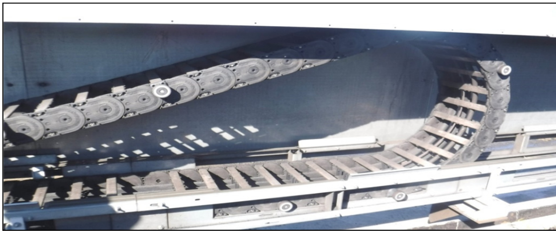
Fig. 3. A cable chain assembly that allows you to carry out reciprocating movements «Staker» along the working area of the coal warehouse
