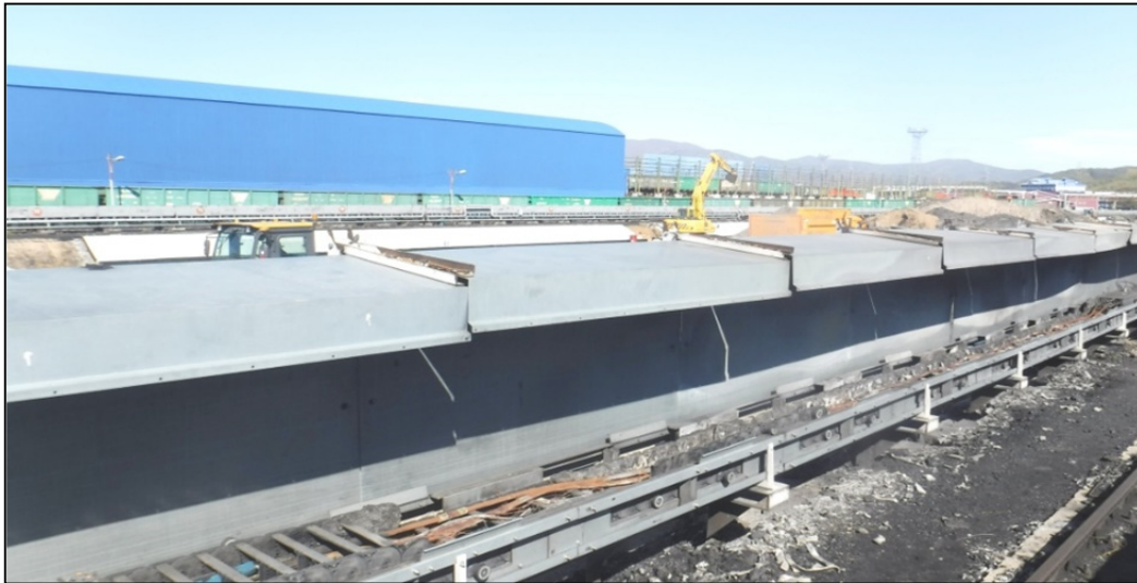
Fig. 4. Thermal damage to the section of the cable chain of the system dust suppression «Stacker»
