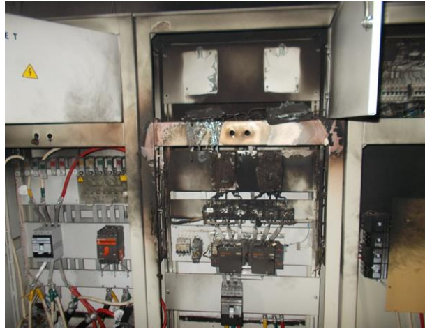
Fig. 3. Bad Consequences of a large short circuit in a building's electrical panel
